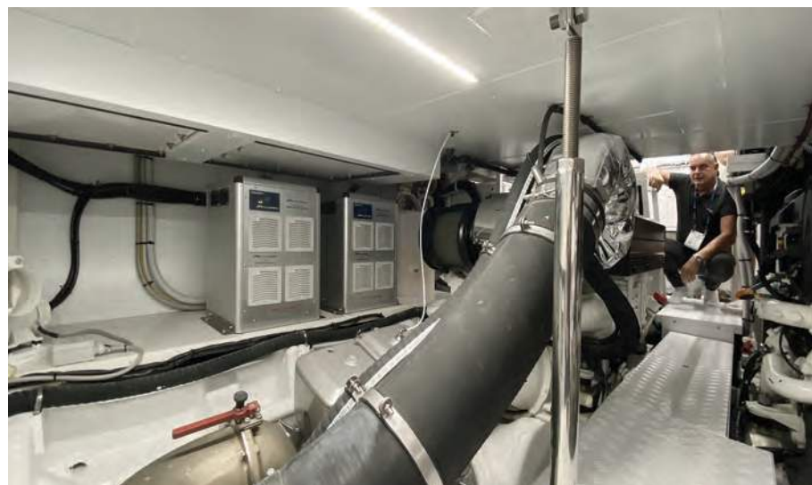
YACHT ISO-BOOST 2x25kW installed on a Sanlorenzo Yachts SX88
